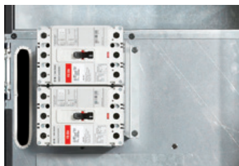
Additional subfeed with aux and shunt trip
